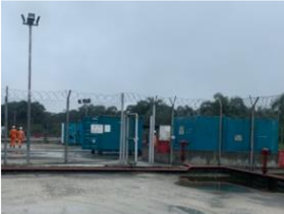
Site Power Generators
