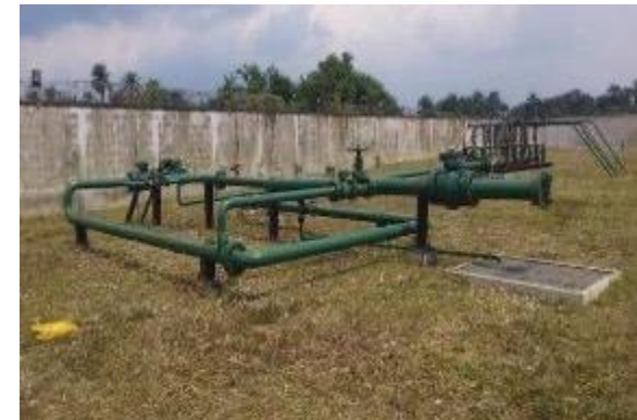
Oza Manifold & Pipeline Launcher
