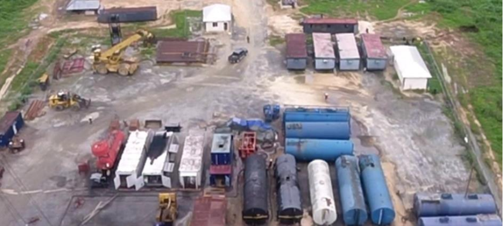
Oil storage tanks in place
