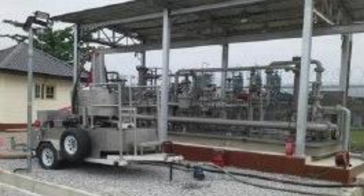
Lease Automatic Custody Transfer Unit #1
