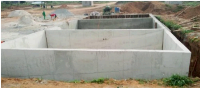
Oza-1 water holding tanks
